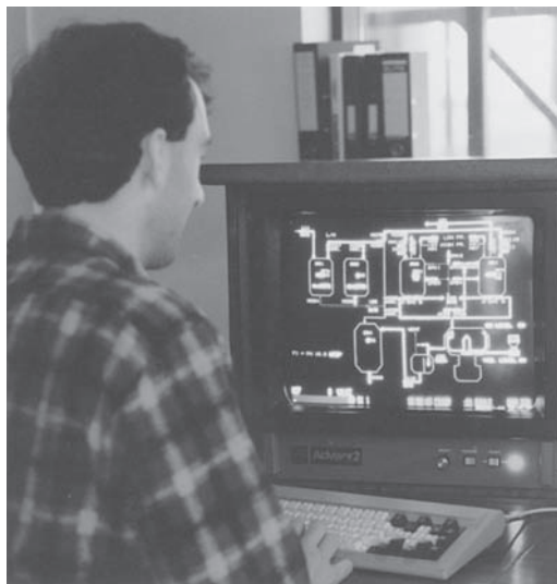
FIGURE 3.1 Example of computer use in the pharmaceutical industry. The machine shown is an Allen Bradley Advisor 21 operator interface. This allows the plant operator to communicate with the main programmable logical controller. The Advisor 21 gives a constant real-time update of the process on a series of screens and allows an operator to perform programmed operations at the push of a button. (Courtesy of Elan Corporation, plc.)
