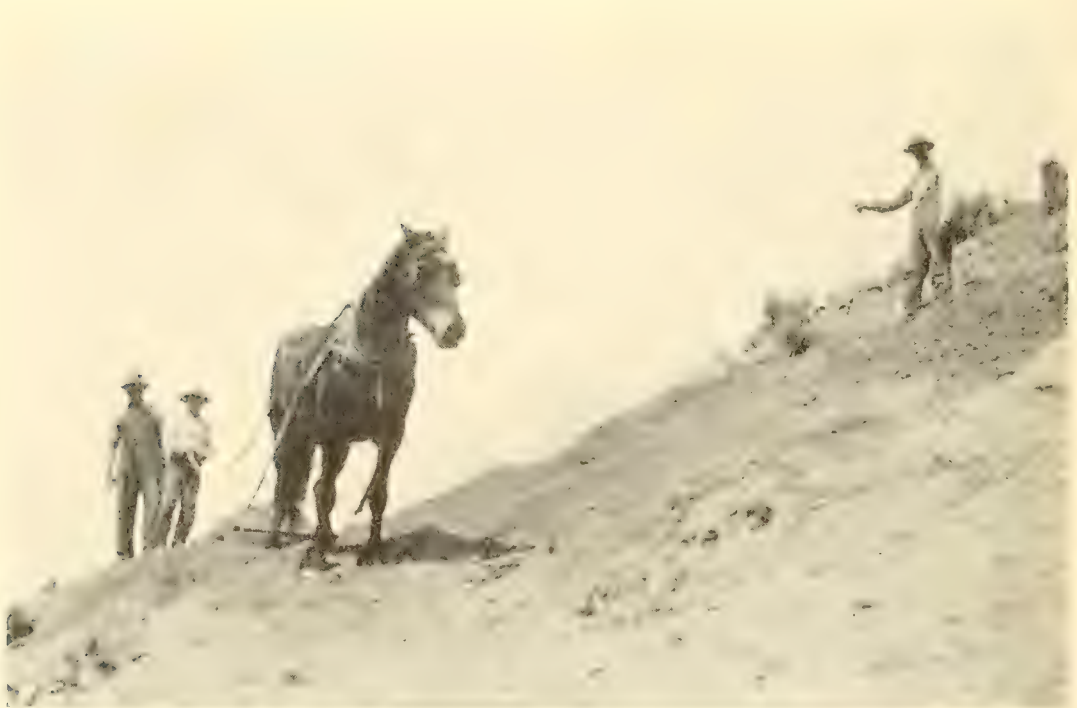
FIG. 36.—Starting the stripping above the bone layer. (Photograph by N. H. Boss.)
