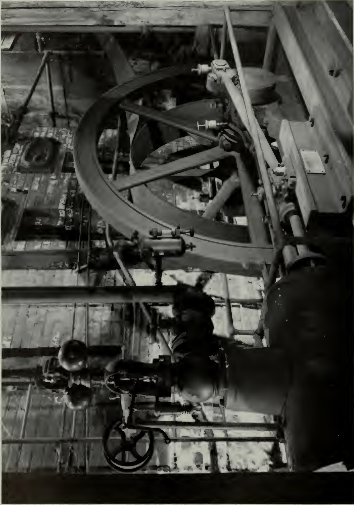
ANOTHER SCENE IN THE EBT SHOPS. Steam from two 100-horsepower Babcock & Wilcox boilers powered this stationary steam engine, which in turn was belted directly to the main shaft that ran all the overhead-belt-driven machinery in the railroad's shop complex. The 12" x 20" stationary engine, which operated at 112 revolutions per minute, was assembled by the EBT workers, who used parts from an undetermined source.
