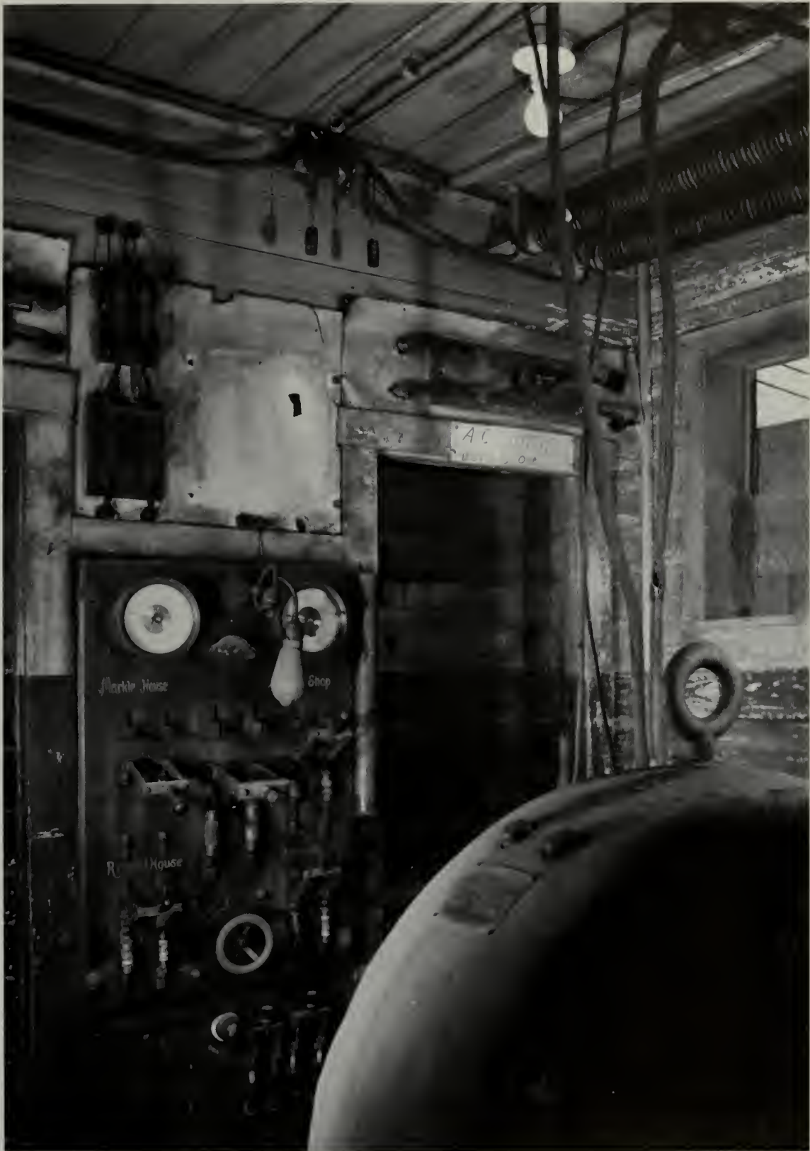
IN THE FOREGROUND, PART OF A 17.6-KILOWATT WESTINGHOUSE DIRECT CURRENT GENERATOR. From a room off the shop boiler area, this generator supplied electrical power for lighting the shops, the roundhouse, and other areas. Also shown is the distribution switch panel.
